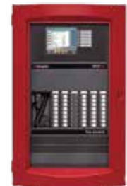
Fire Control Panel
